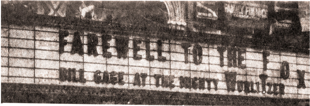
Workmen starting to tear down the marquee of the Fox Theater on Flatbush Avenue, Brooklyn
