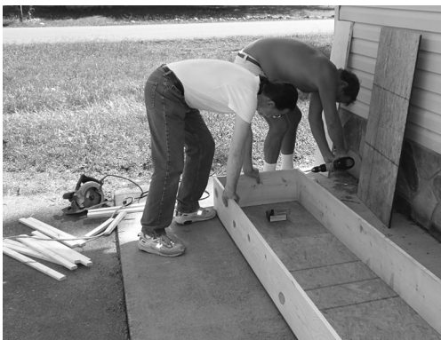
Phil Hargiss and Dave Luttinen build crates on-site to hold the donated pipework
