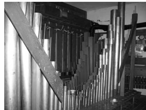
Pipework in the understage chamber
